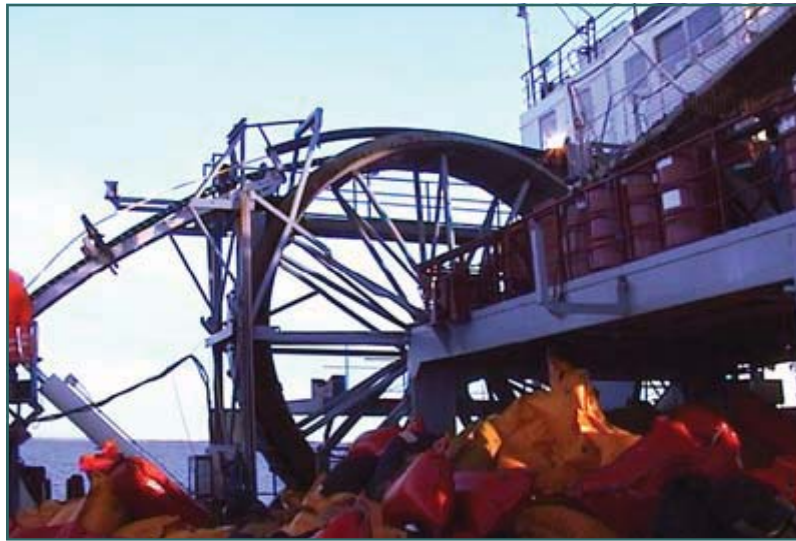
The laying method used by JD-Contractor ApS is to have the cable hanging in a catenary curve from C/B Henry P. Lading to the seabed.
